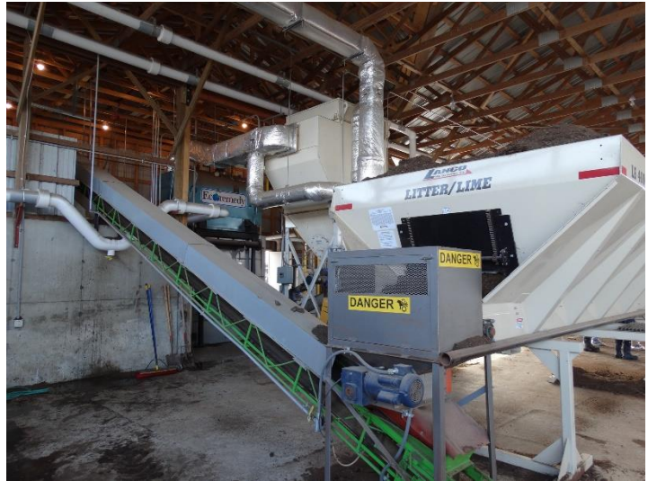
Figure A-15-1. Combustion system at poultry operation. Photo: Livestock and Poultry Environmental Learning Center (LPELC)
