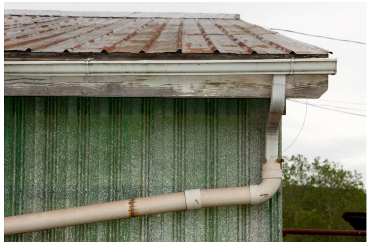
Figure A-7-1. Gutters, or roof runoff structures, can divert precipitation away from areas where animals and manure are present, which keeps the runoff water clean. Photo: USDA NRCS
