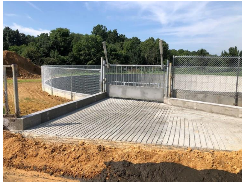
Chester Conservation District Manure storage facility with safety fencing and scrape in (90' diameter x 12' depth) in Knight Run Watershed, Octoraro Creek Reservoir (Growing Greener in partnership with NRCS)
