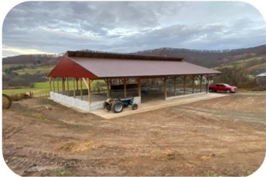
McKean County Conservation District Roofed heavy use area and manure stacking pad for beef operation along Annin Creek (Growing Greener)
